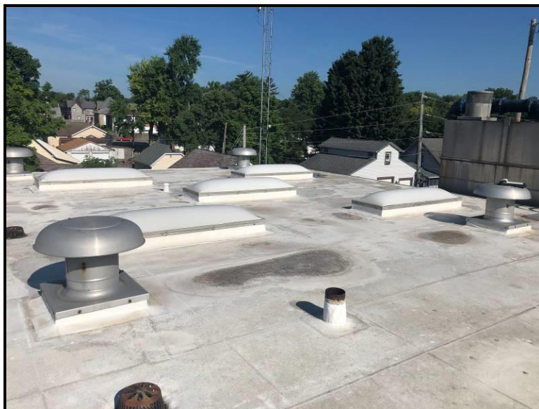
Figure 2-3 Overall view of the upper roof including localized ponding and skylights.
