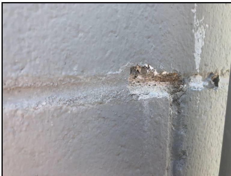
Figure 2-4 Failed repointed mortar joint adjacent to the intermediate roof deck.
