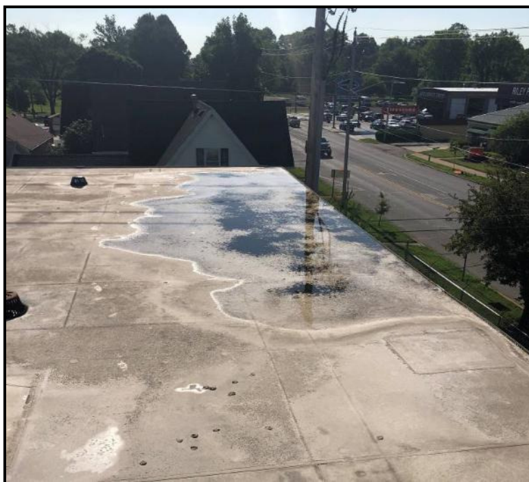
Figure 2-1 Representative ponding in the South East corner of the roof.
