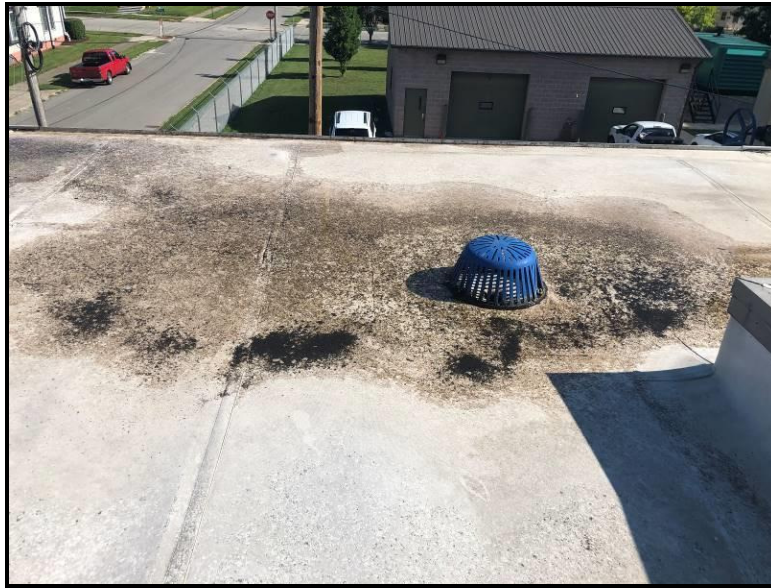
Figure 2-2 Ponding around an improperly installed roof drain.
